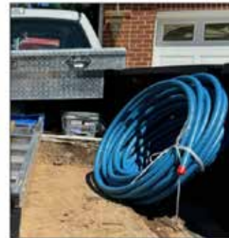
Figure 9.1 PEX Tubing Stored Outdoors
